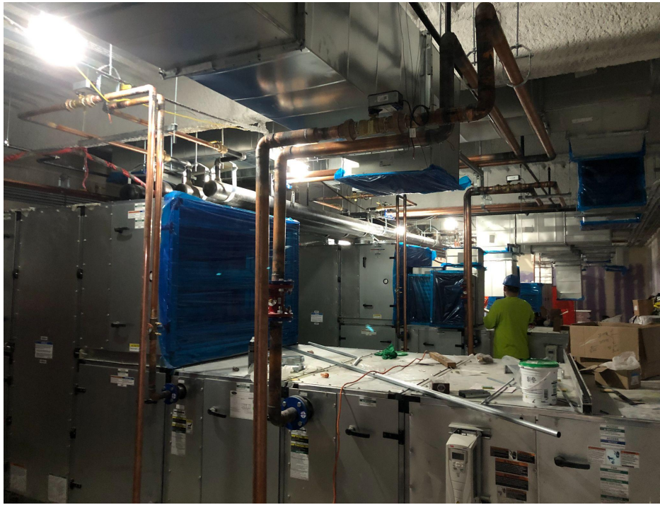
Mechanical Room in Academic Area
